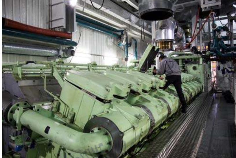
Figure 4.6 Commissioning 18V48/60 with two stage turbocharger
