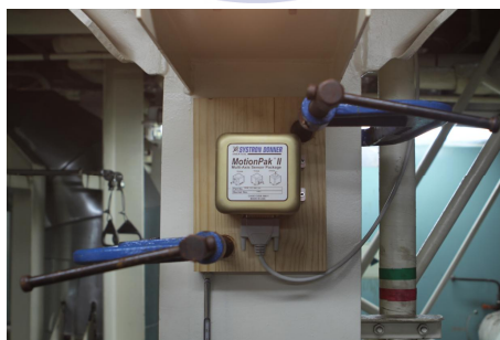
Fig. 3-7 MotionPak installed in the engine room
