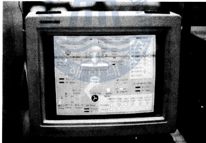
Photo. 3 Maneuvering Window of Press. & Level control of Aux. Boiler
