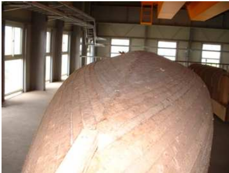
Fig. 14 Troubles in connecting by the strips
