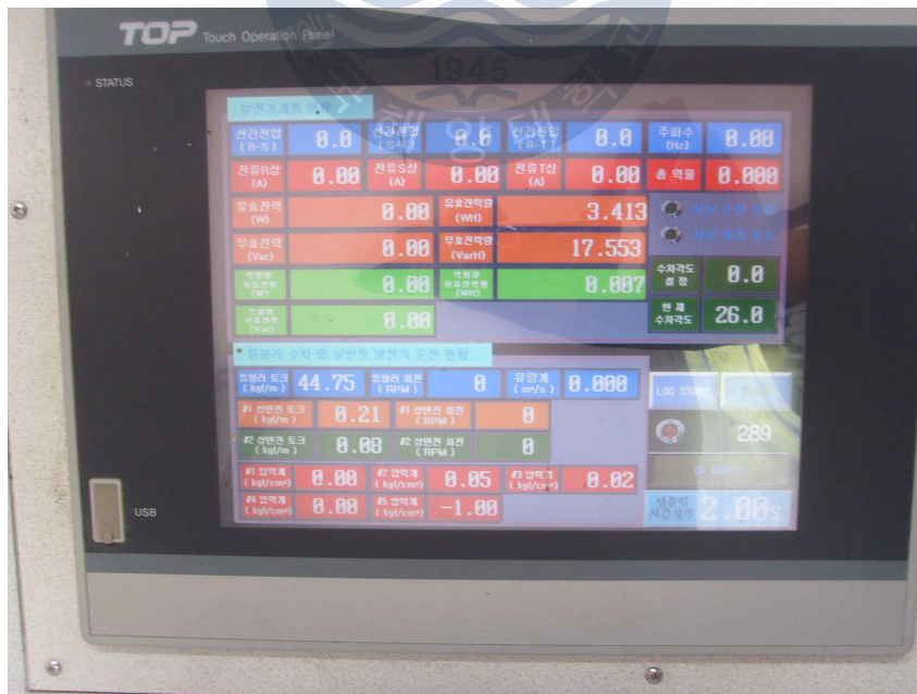
Fig. 3.19 Operating condition of counter-rotating tubular type turbine
