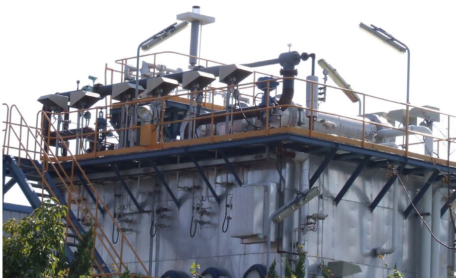
Photo 4.2 Experimental plant of MED-TVC pilot plant
