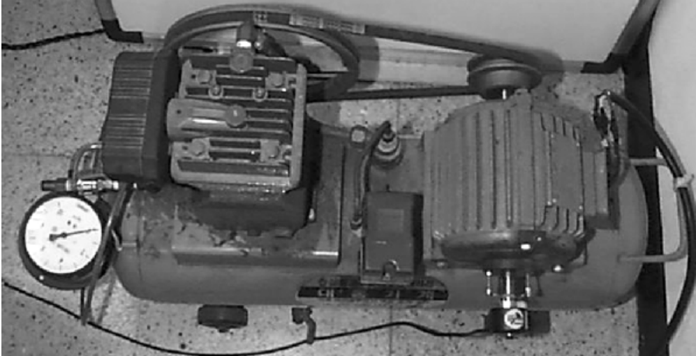
Fig. 5-4 Photograph of the air compressor
